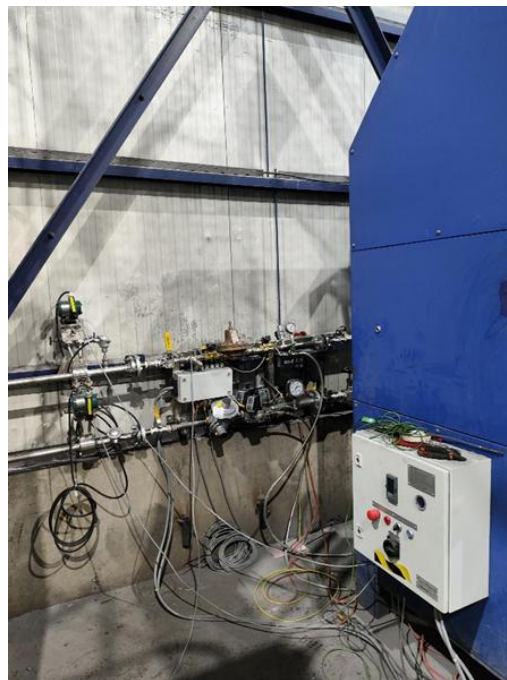
Figure 3: Flow skid mounted on the wall and the control cabinet on the hydraulic cover
