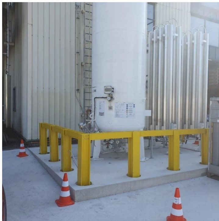
Figure 97: Oxygen tank and evaporator
