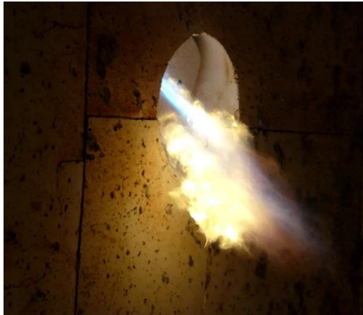
Figure 100: Flame before correction of burner position
