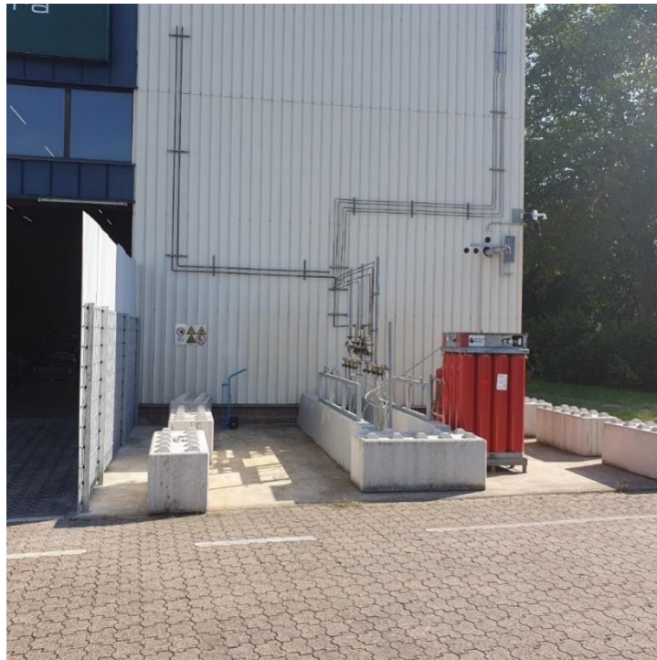
Figure 98: Hydrogen cylinder rack
