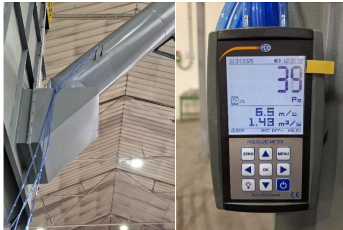
Figure 29: Details of installed pitot tubes and register
