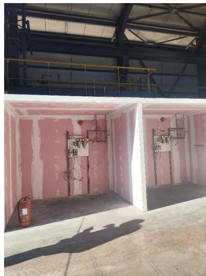
Figure 1: Safety walls for hydrogen and oxygen bundles
