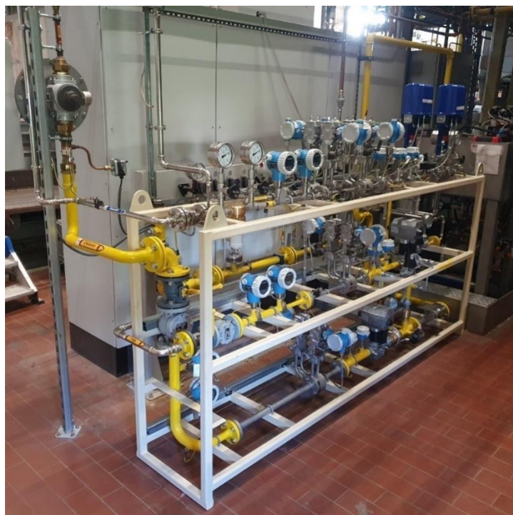
Figure 99: Skid for hydrogen and natural gas supply
