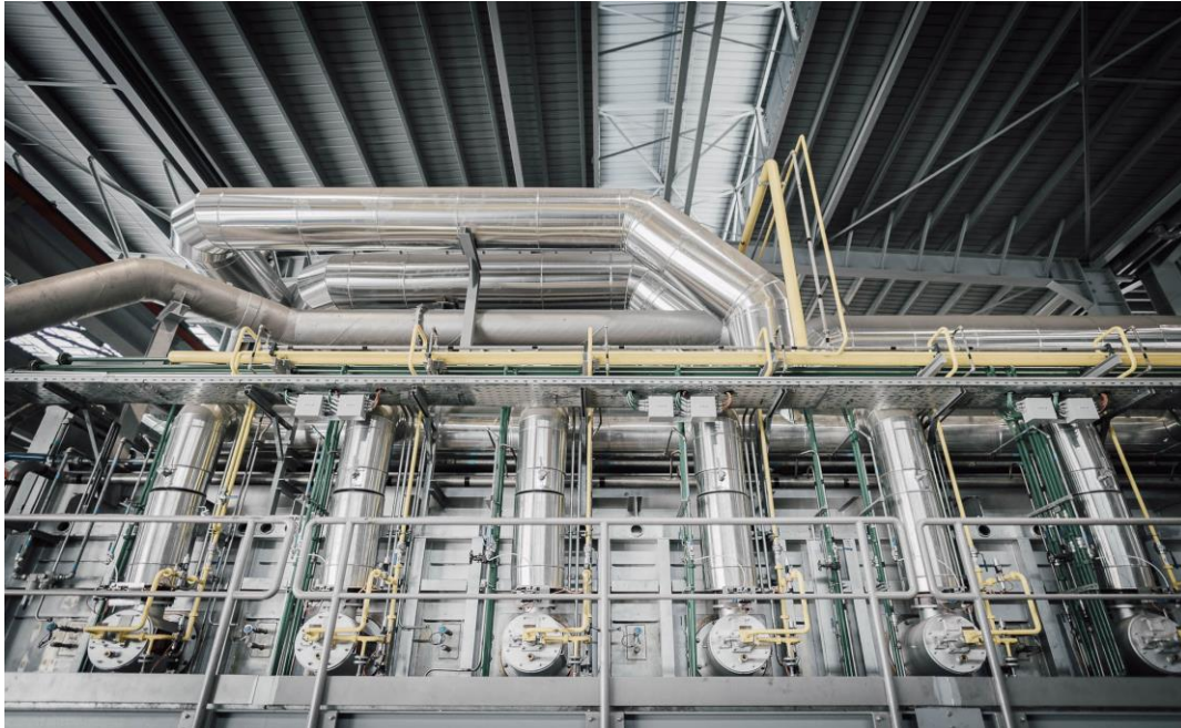
Figure 105 - Scale free furnace sidewall Burners
