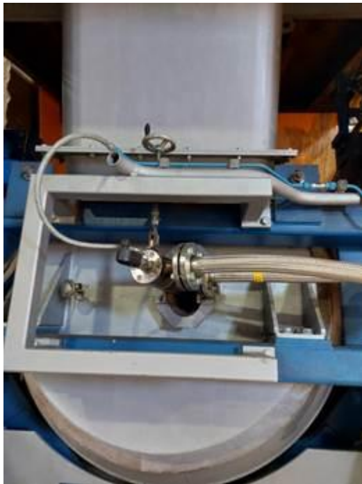
Figure 3: J Burner at furnace's door.
