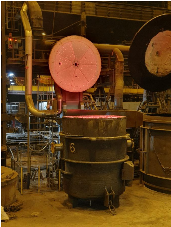
Figure 149. Photo of the ladle heater roughly one minute after shutdown.
