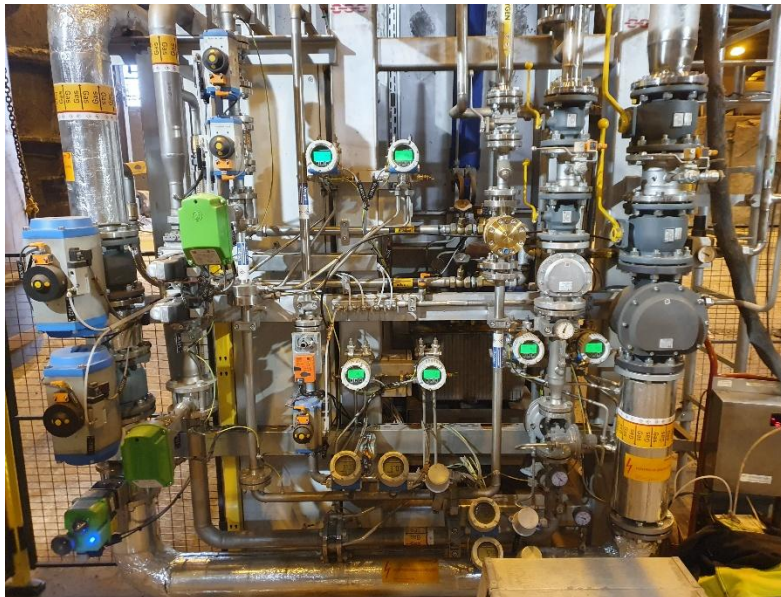
Figure 129. Photo of piping and instrumentation on the rear side of the ladle heater.
