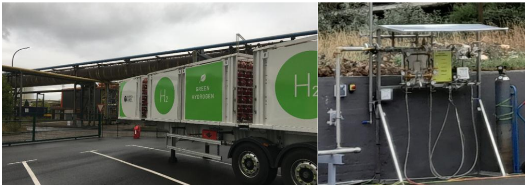
Figure 189. Hydrogen supply and decompression station at AMI.
