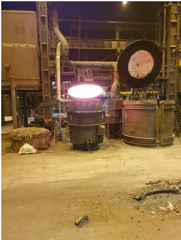
Figure 148. Photo of the lid of the ladle heater opening at the end of the hydrogen heating test.
