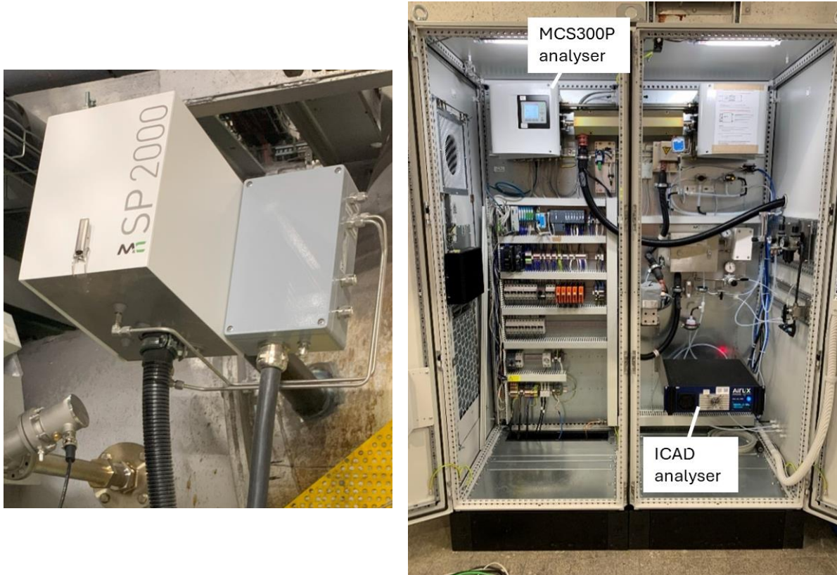
Figure 13: Installed MCS300P analysing system left: Sample gas probe, right: analysing cabinet with MCS300P and ICAD analyser
