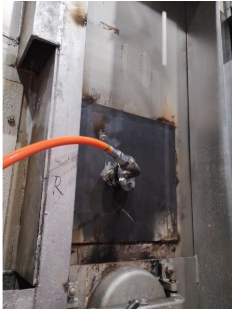
Figure 6: Installed OES measurement head and guide tube.
