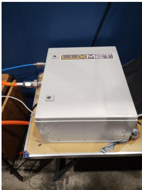
Figure 7: Installed OES equipment cabinet.
