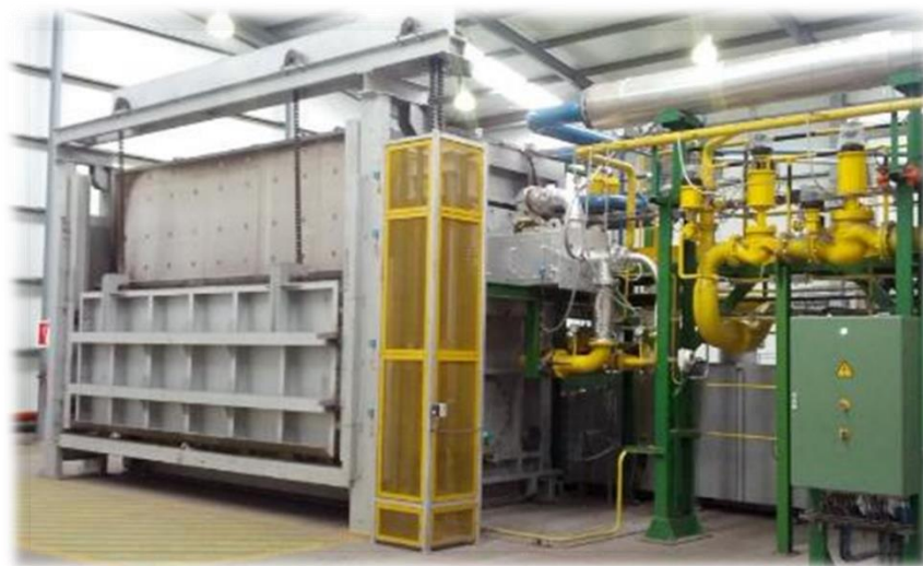
Figure 4. AMI direct furnace testing facility.
